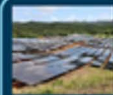
Palau Solar and BESS, first foray outside the Philippines, the largest solar and battery energy storage in the Western Pacific. Energized in December 2023.
